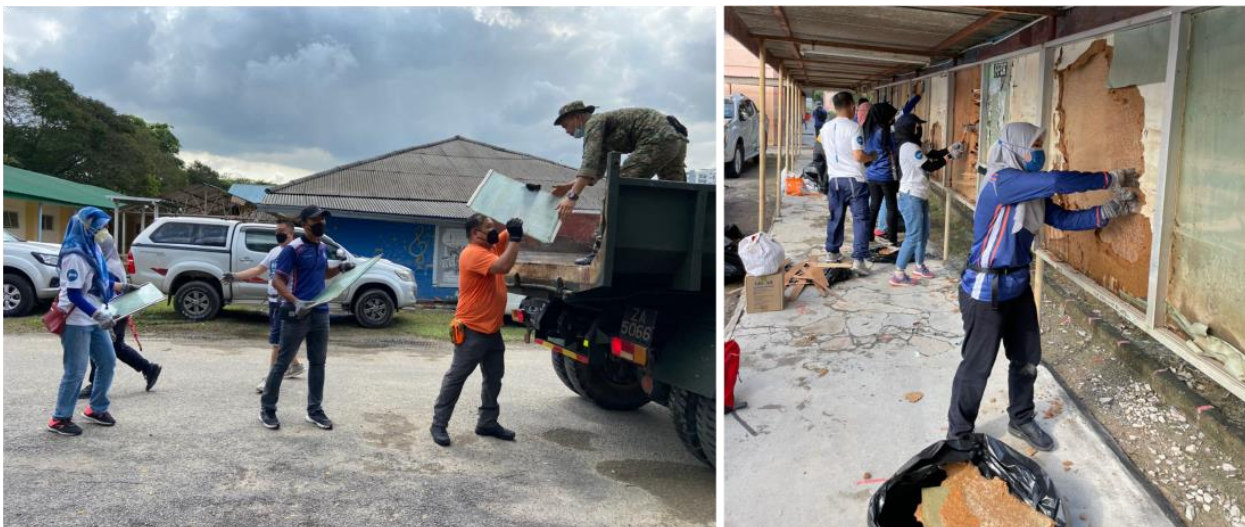
Left: Clearing away all debris . Right: Dismantling the damaged notice board process.
